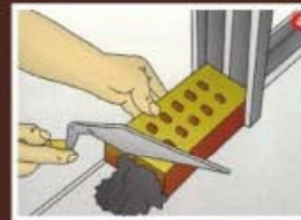
Begin brickwork by laying the bricks into the rebate behind the back of the metal door frame.
